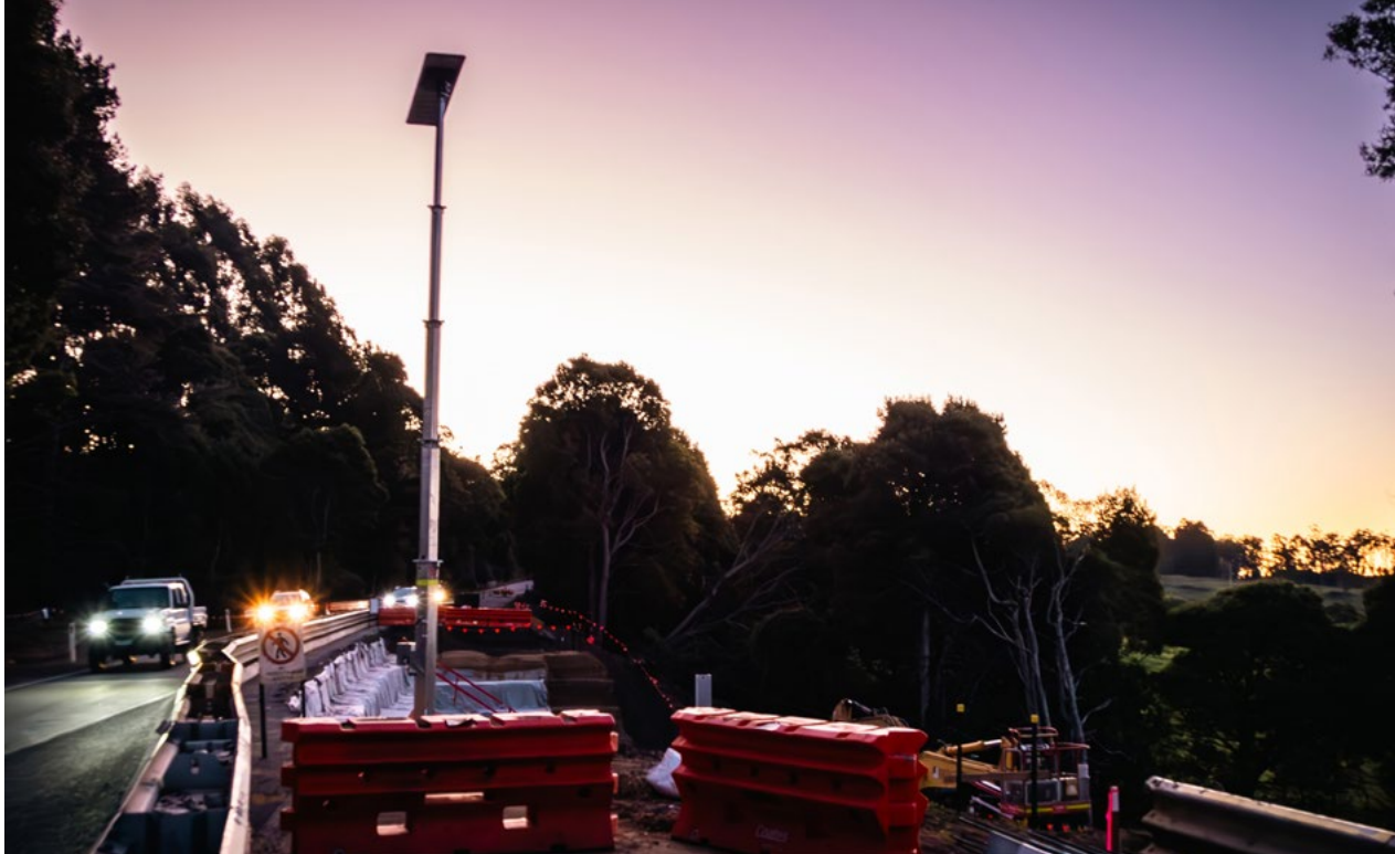
Blade Solar Light deployed at a Fulton Hogan site, Carrarung, Victoria.
